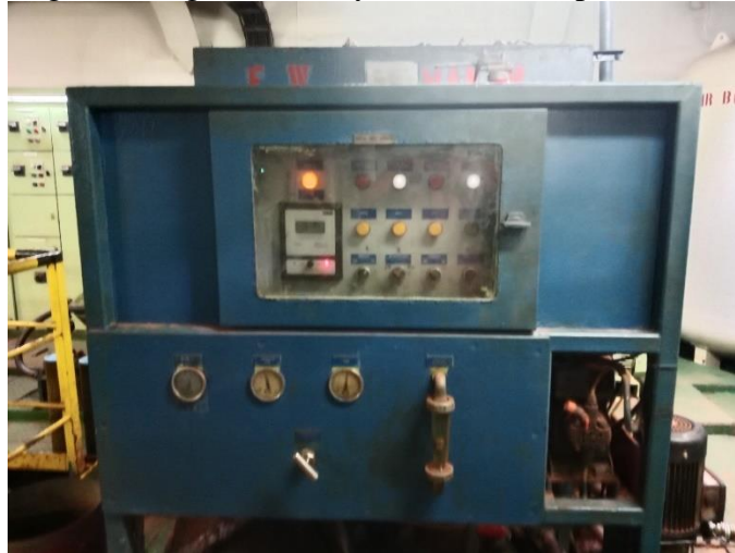
Gambar: 7. Panel FWM STS RO SW-10T
