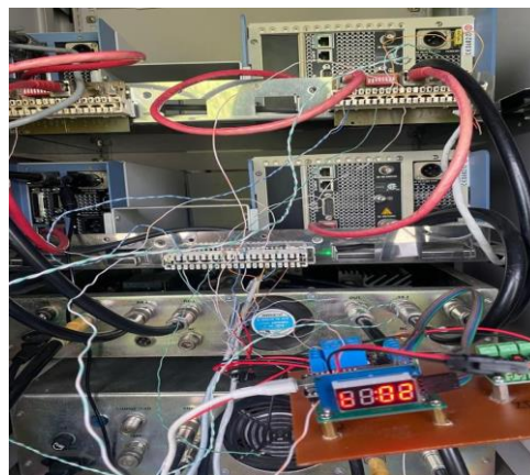
Gambar 7. Rancangan Changeover Otomatis Diimplementasikan di Transmitter VHF Air To Ground R&S SU4200
